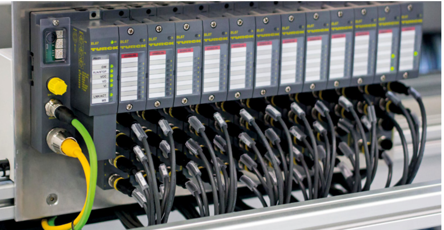
Turck's BL67 I/O system processes and controls the signals of the plant and communicates with the IPC via Modbus TCP
