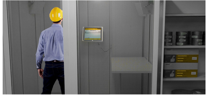
Each Unmanned Store will have a separate Read Area to ensure all products have been registered
