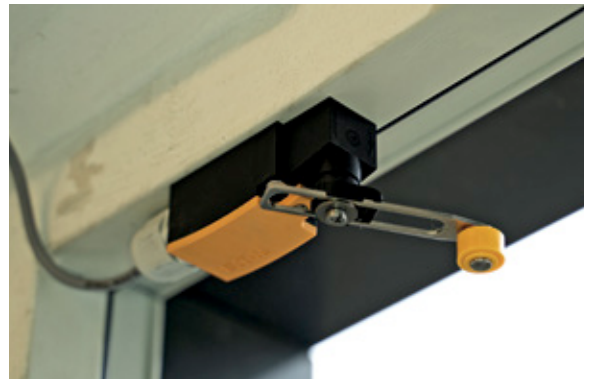
Insecure door contacts or roller switches that were costly to install were not considered for retrofitting the cabinet guarding system
