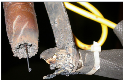
Typical damage from MIG welding
